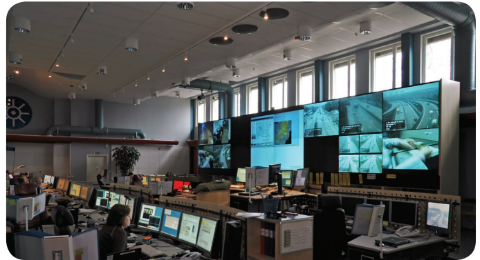
Trafik Stockholm - Regional Traffic Control Centre
